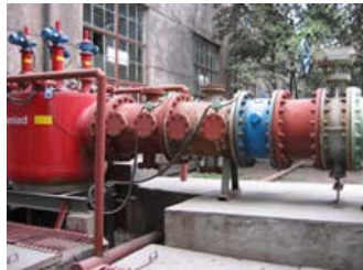
Ultrasonic descaling & anti-scaling for dust-removal system in steel mill.
