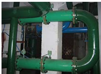
Ultrasonic descaling & anti-scaling for oxygen compressor in ethylene plant.
