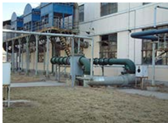
Ultrasonic descaling & anti-scaling for heat exchanger in petrochemical plant.
